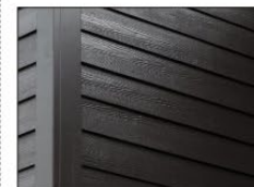
Primary Wall Material - Black cladding on select properties as shown on elevations
